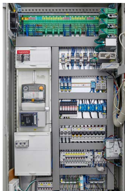
A look inside the control cabinet: Central controller with communication modules
